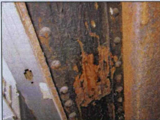
Photo 1. Coal tar coating on column at Location 1.
