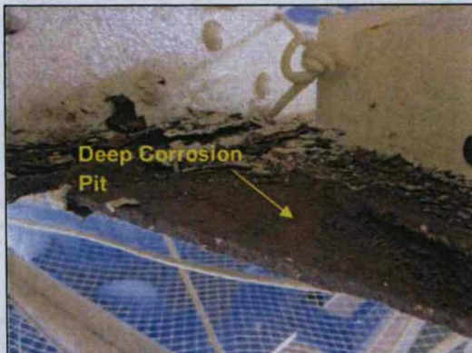
Photo 19. Bottom chord gusset plate with moderate pitting.
