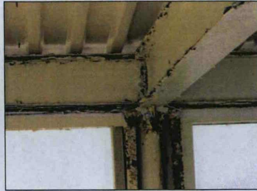
Photo 28. Typical exfoliation of beam flanges at connection point between top longitudinal and transverse beams.
