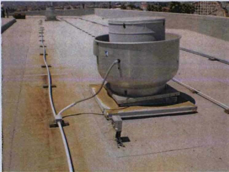
Figure 6. Exhaust Fan (Typical of 6)
