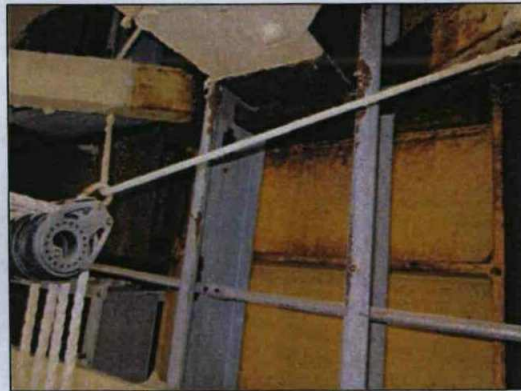
Photo 2. Yellow coating on post 1987 retrofit moment frame with spot blistering.
