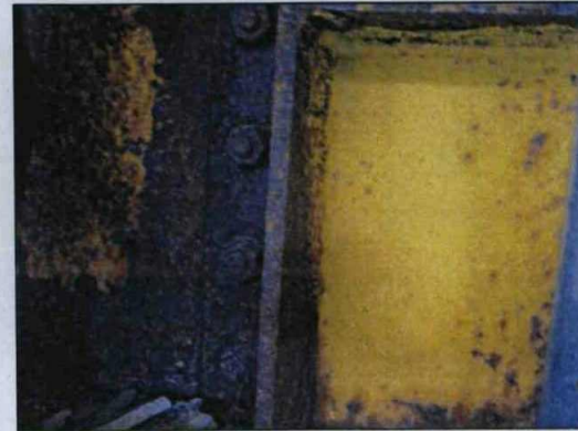
Photo 10. Intermediate moment frame connection at Location 4 with pitted beam.
