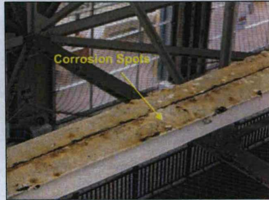
Photo 18. Corrosion spots on top chord truss members.
