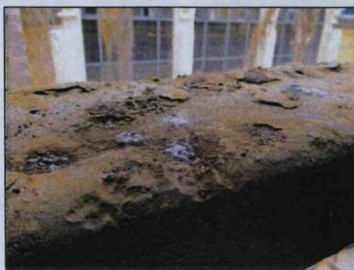
Photo 22. Detail of corrosion nodules on lateral-brace tube after removal of corrosion products (weakened steel).
