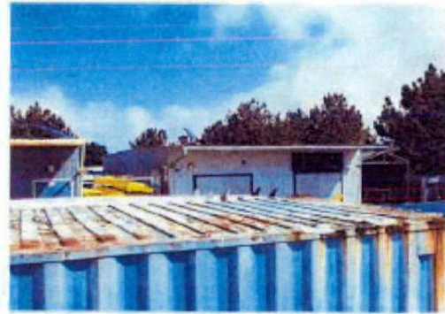
Deteriorating Roof on Storage Container
