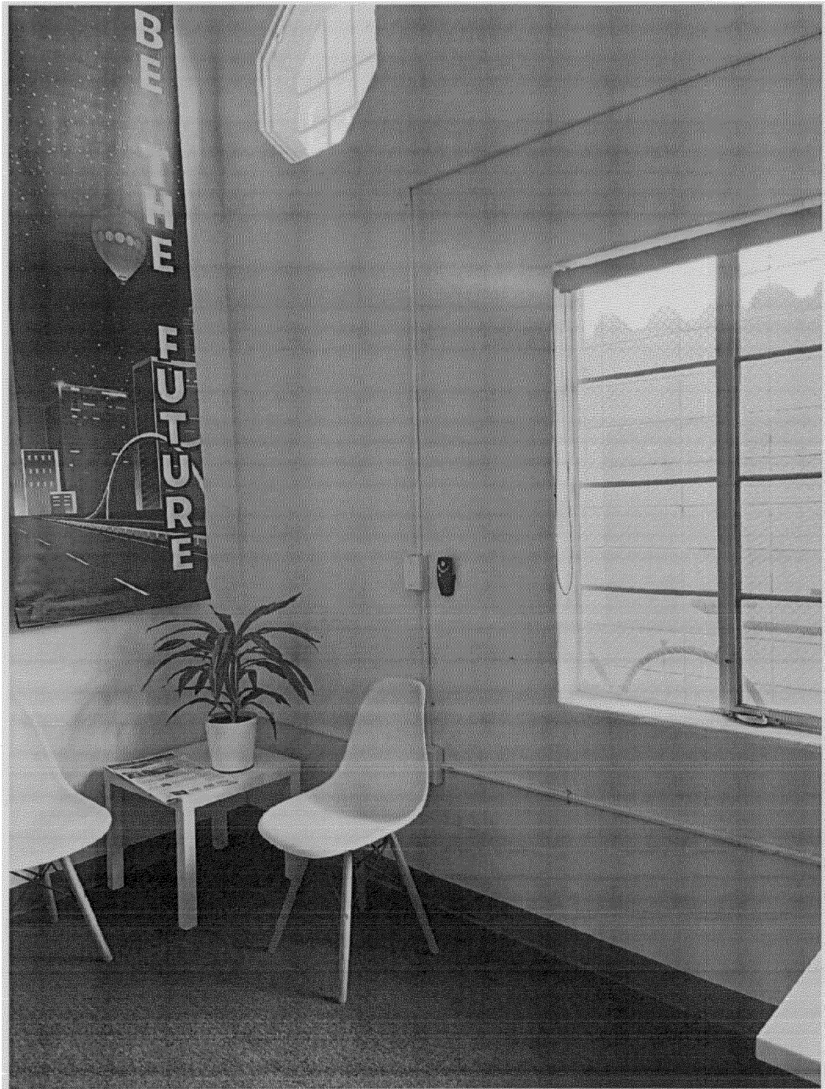
Chairs in Study Room. Window will be replaced.
