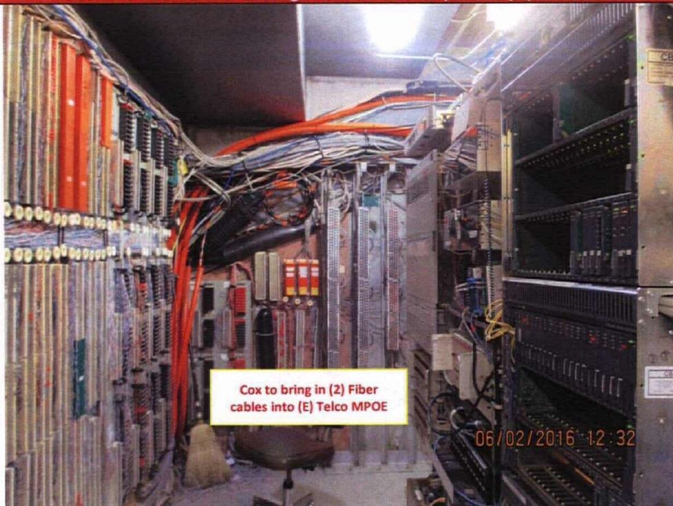
Club Level - Section 21: Existing Telco MPOE in Telephone equipment room
