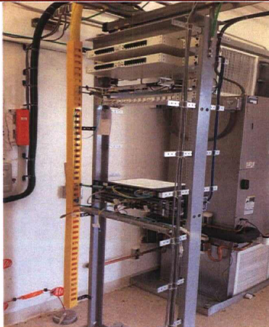
View of (E) Verizon Equipment Cabinet/Rack
