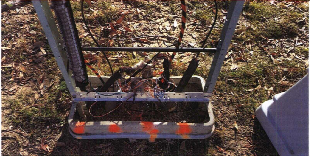
View of (E) Pedestal feeding the MPOE
