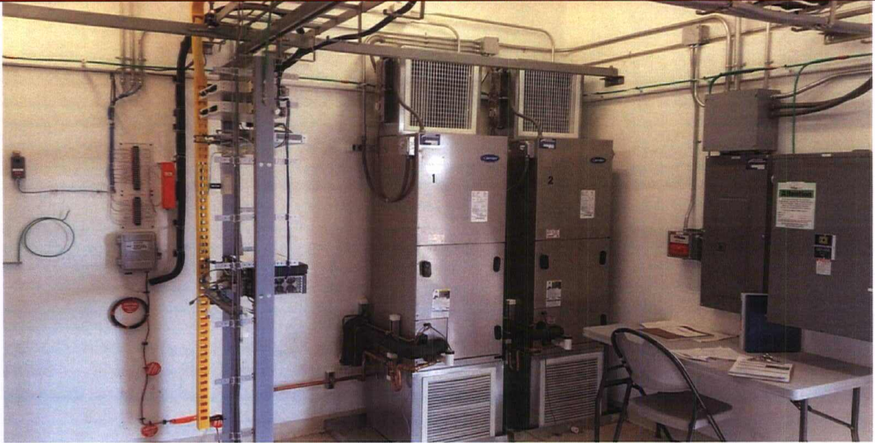
View of Inside Cell Site Panoramic #4
