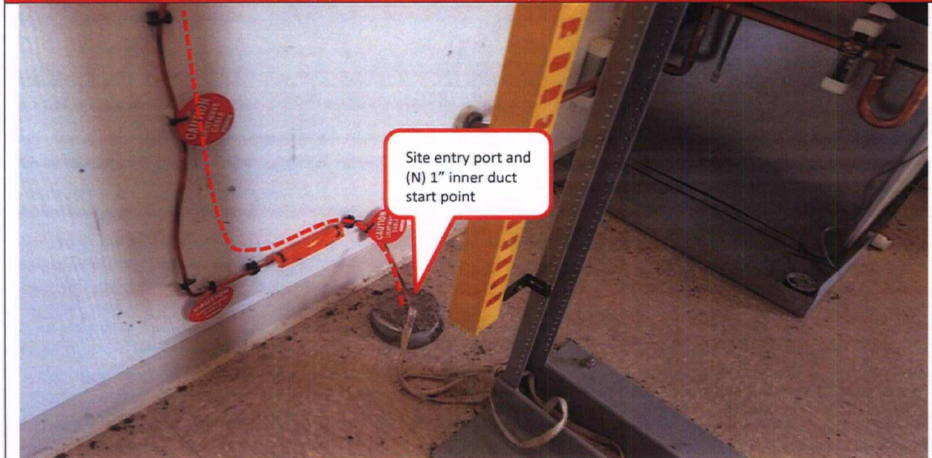
View of (N) Fiber Path from site entry port to VZW toll rack
