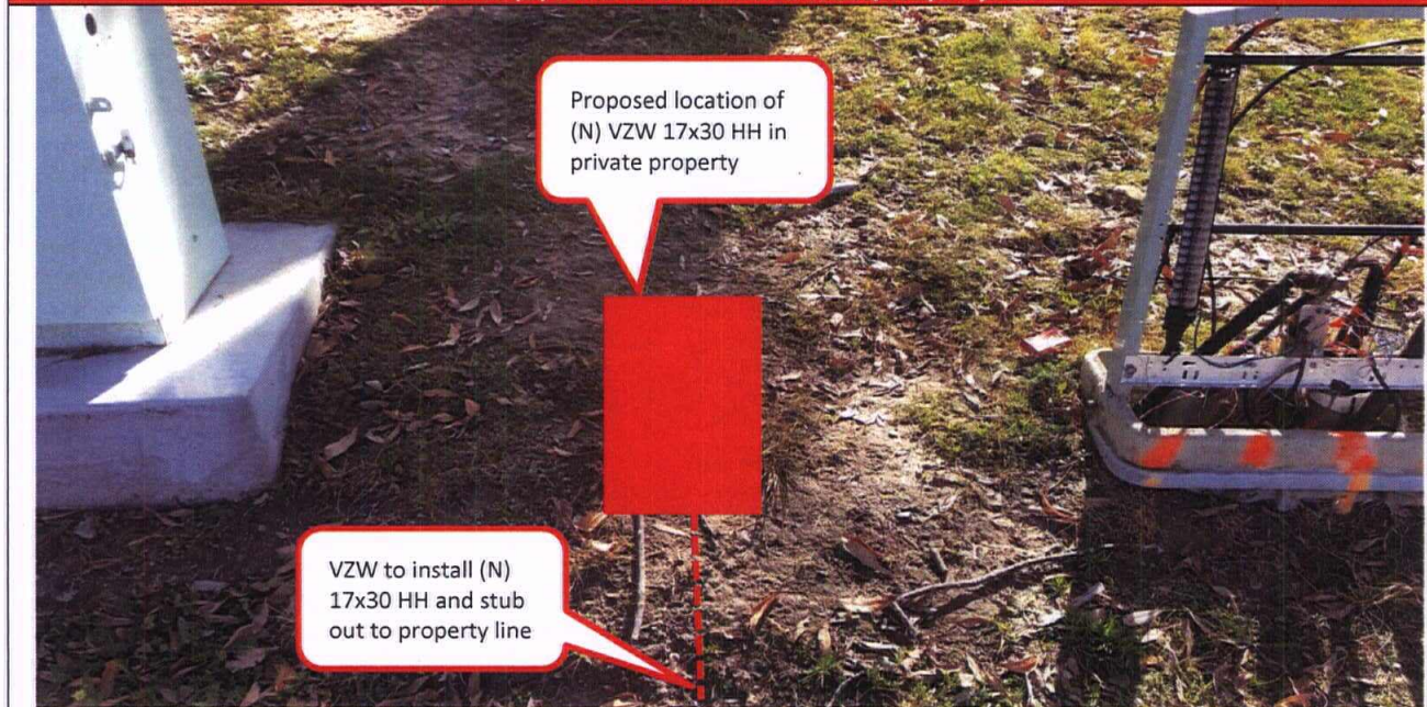
View of (N) Verizon Hand-Hole at ROW/Property Line
