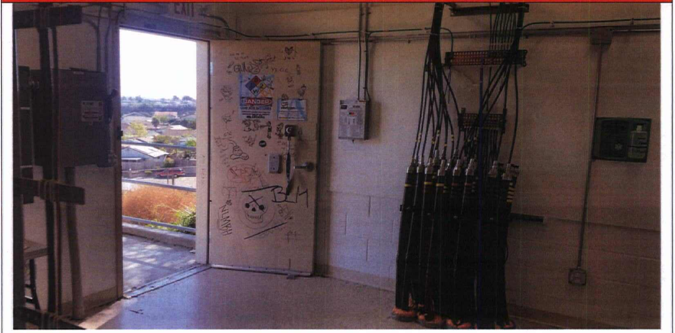
View of Inside Cell Site Panoramic #1
