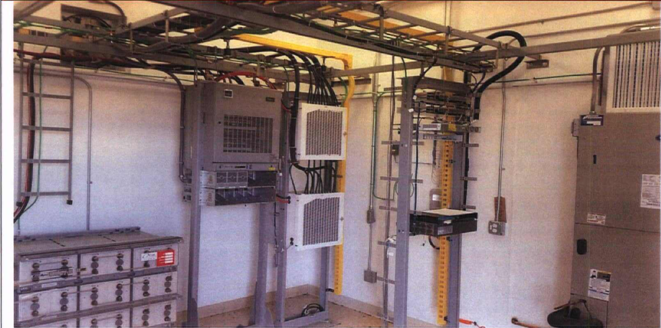
View of Inside Cell Site Panoramic #3
