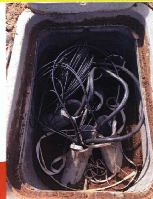
Existing Handhole with Ducts
