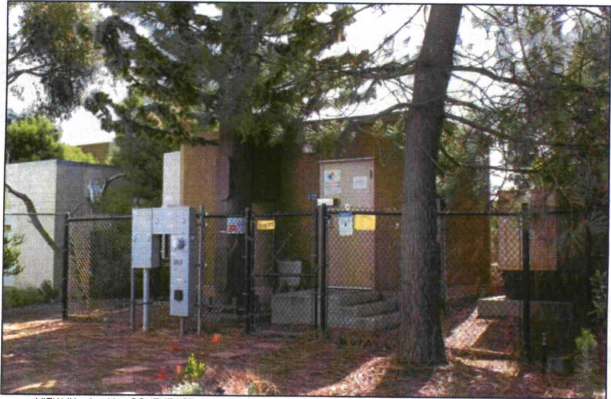
VIEW #1 – Looking SOUTHEAST at existing Verizon equipment shelter and lease area enclosure (to be removed)
